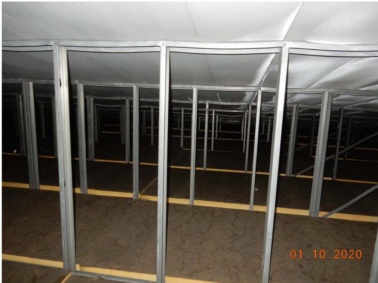
Looking east in attic space in southeast quadrant of school, above classroom wing. Tracks at top of light gage cold formed stud walls are unreinforced and deformed.
