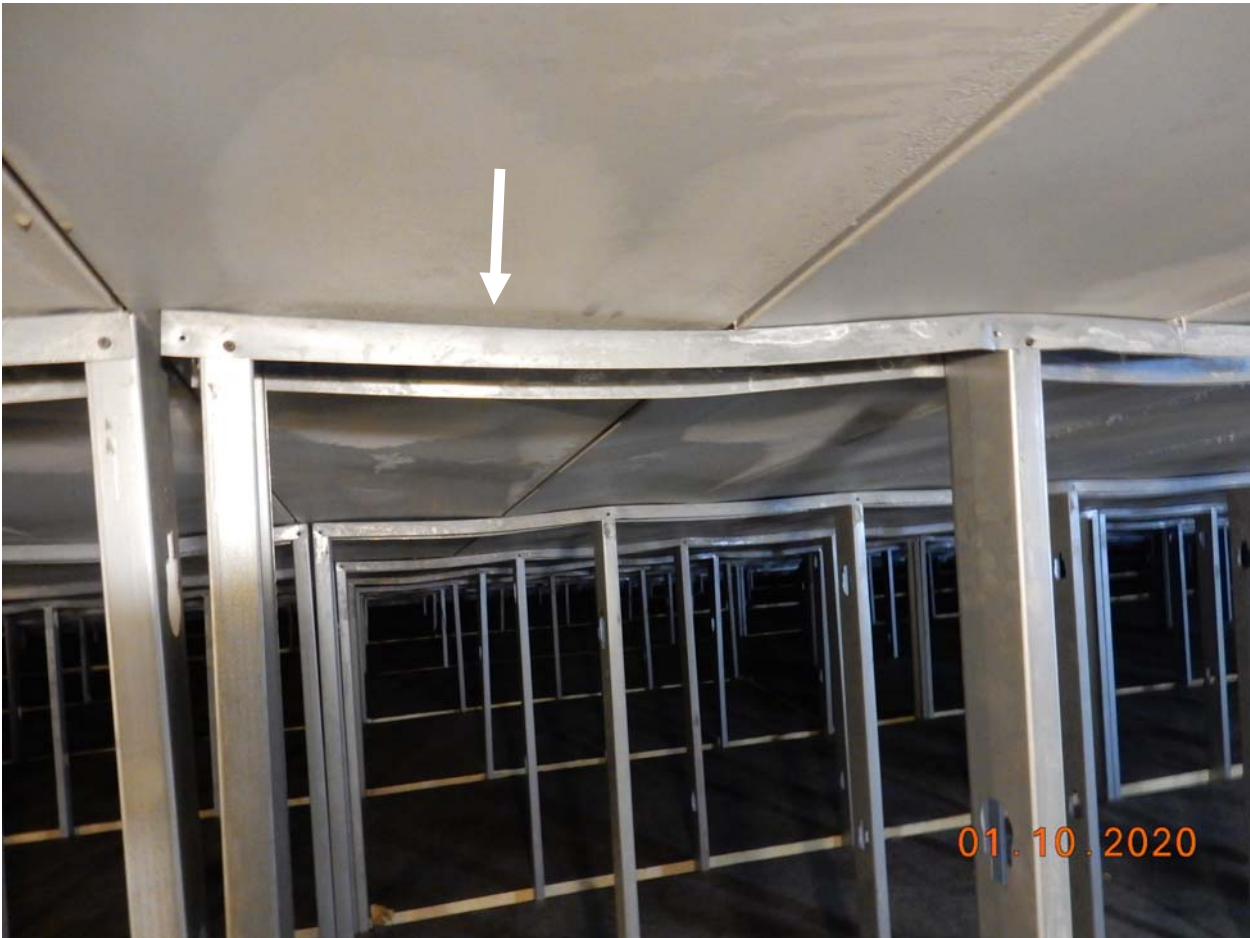
Closer view of deformed tracks at top of studs. Note gap (arrow) between underside of standing seam roofing and top of track.
