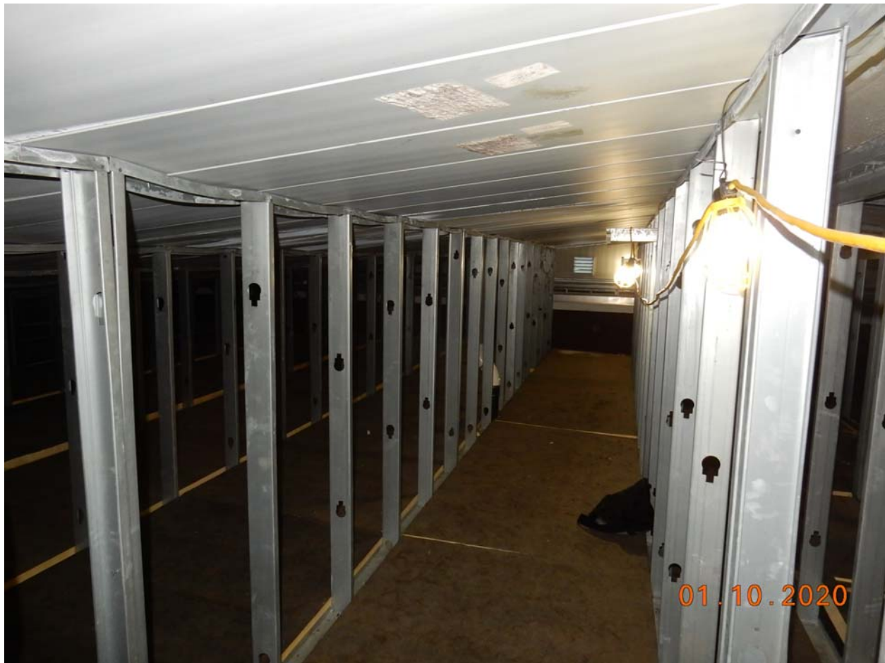
Looking south in attic space in southeast quadrant of school, above classroom wing. Tracks at top of light gage cold formed stud walls are unreinforced and deformed.
