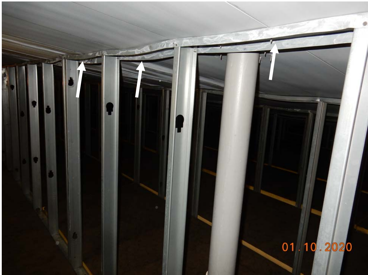
Looking northeast in attic space in southeast quadrant of school, above classroom wing. Track (arrows) at top of light gage cold formed studs is unreinforced and deformed.
